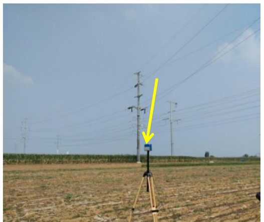
B11: 110kV 蒋观线 48#塔~49#杆塔导线衰减
